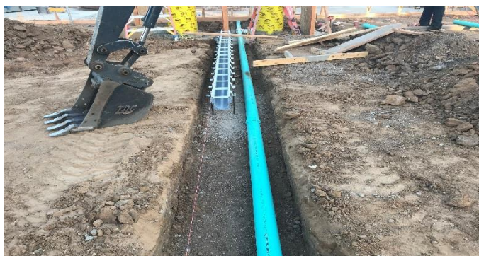
Lunch court trench drains
